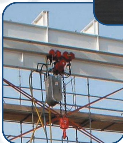
Detail hoist and trolley
